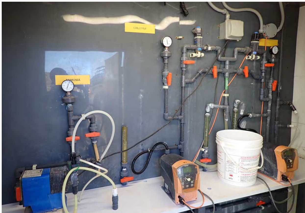
Figure 5.4 Water Quality Sampling Station at Vine Street Filtration Plant
